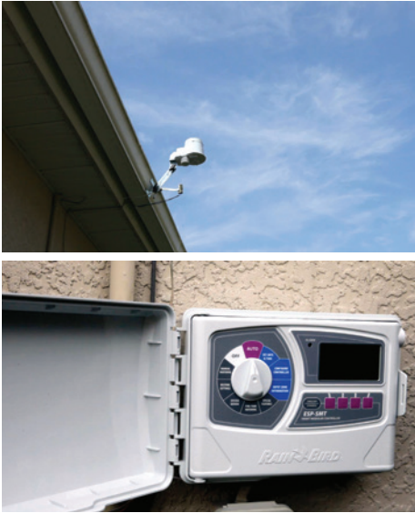
Figure 1. The components of a Rain Bird ESP-SMT include A) the irrigation controller that replaces the timer and B) an independent weather station that replaces the rain sensor (still pictured) on the roof eave.
