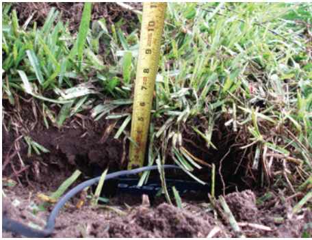
Figure 3. The Baseline Watertec S100 soil moisture sensor was buried in a trench at a 6 inch depth chosen by the irrigation contractor.
