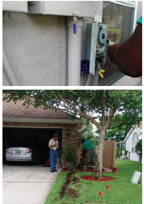
Figure 2. The Baseline Watertec S100 soil moisture sensor was A) buried in the ground and the B) sensor controller was added to the current timer to bypass irrigation events when the soil was too wet.
