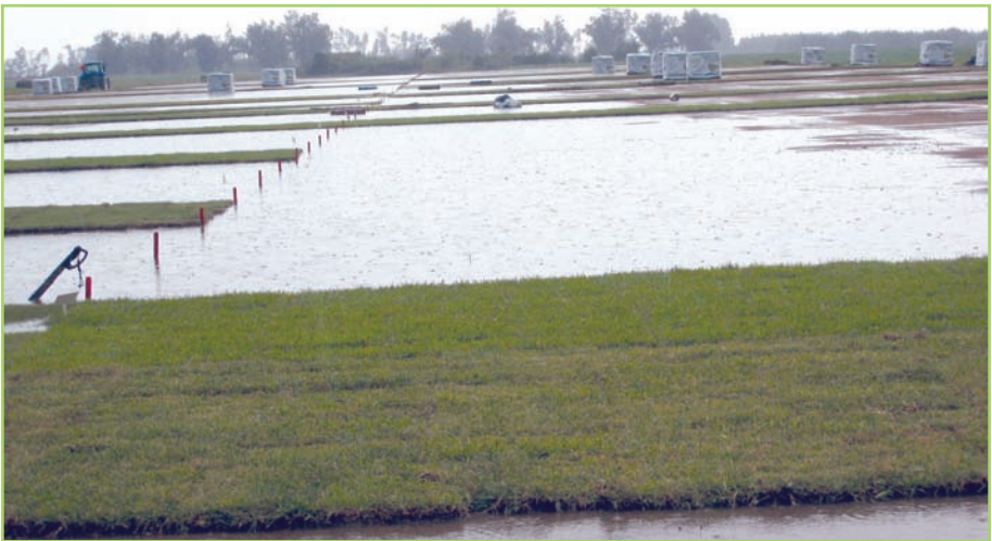
Fig. 2. The subgrade was laser-leveled and shaped to provide 5" drop from the outside inward to ensure all surface water flows to the center as evidenced during the rain event.
